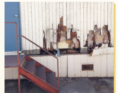
Leaky roofs and walls need repairs ▲
