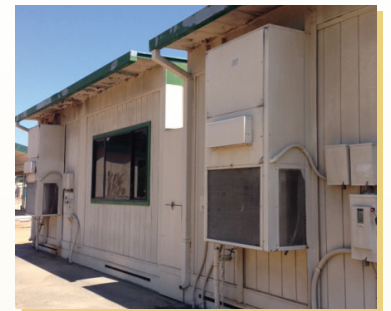
Aging air conditioning systems require updates ▲
